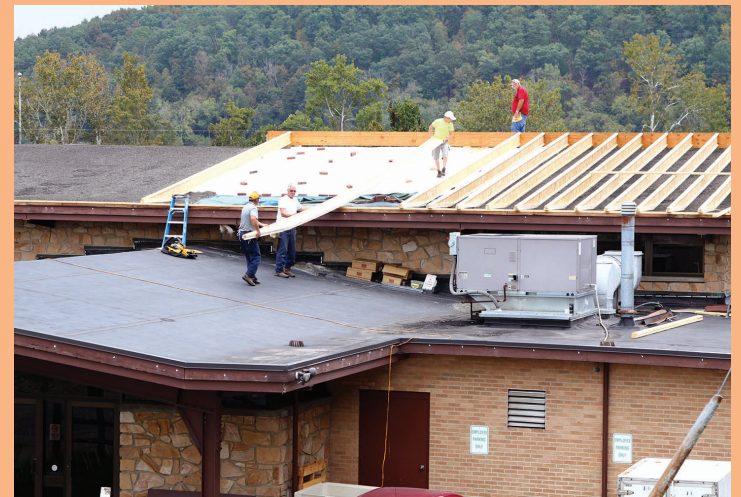
WVDA Building and Grounds staff work to put a new roof on the dining hall at Cedar Lakes Conference Center, part of ongoing efforts to prepare the facility for expanded educational and conference events in the future.
